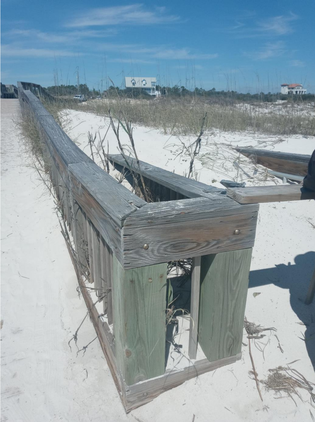
Figure 2: Mobile Street Boardwalk wheelchair ramp (right) completely overtaken by the dunes.
