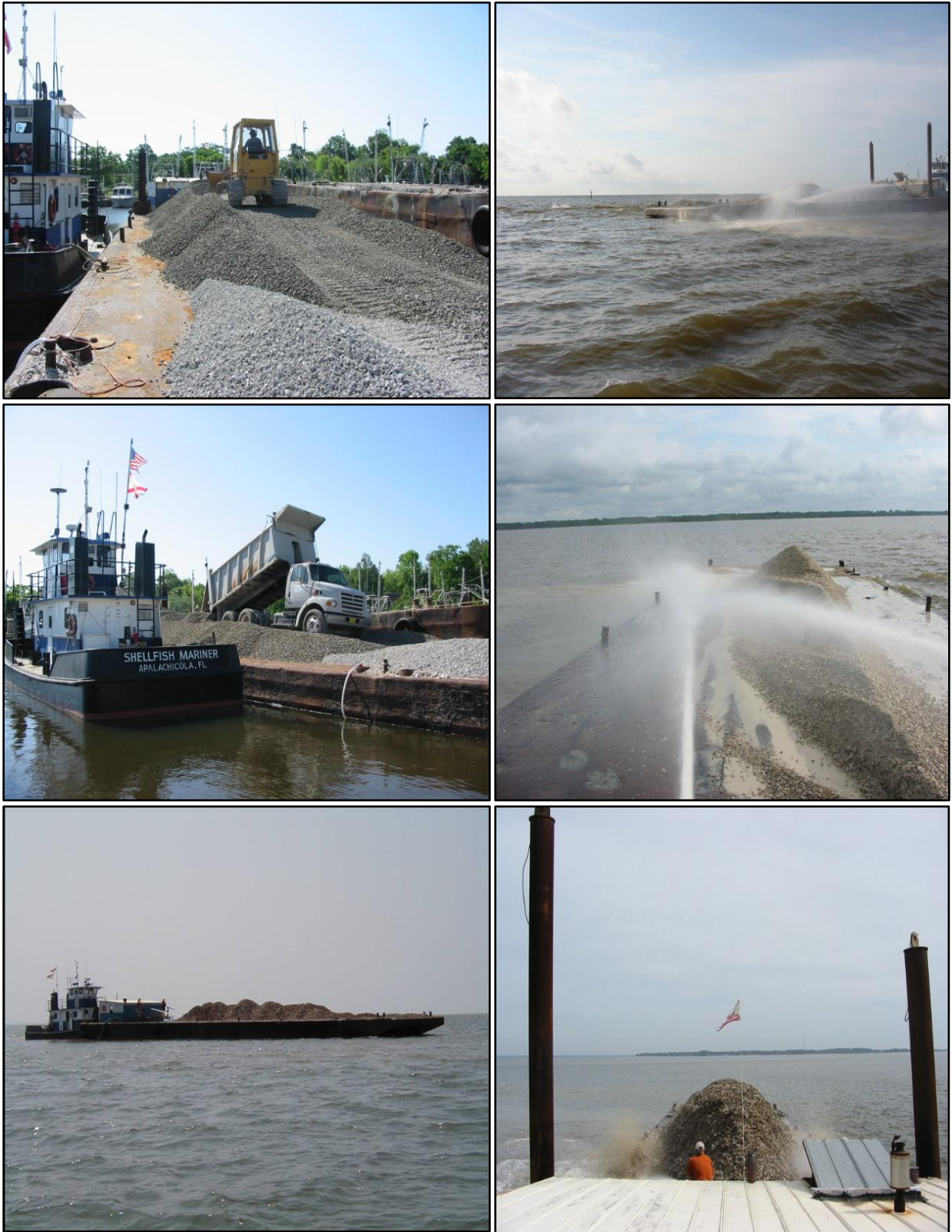
Figure 12-55. Examples of cultch loading and transportation (right images) and offloading using water cannon (left images).
