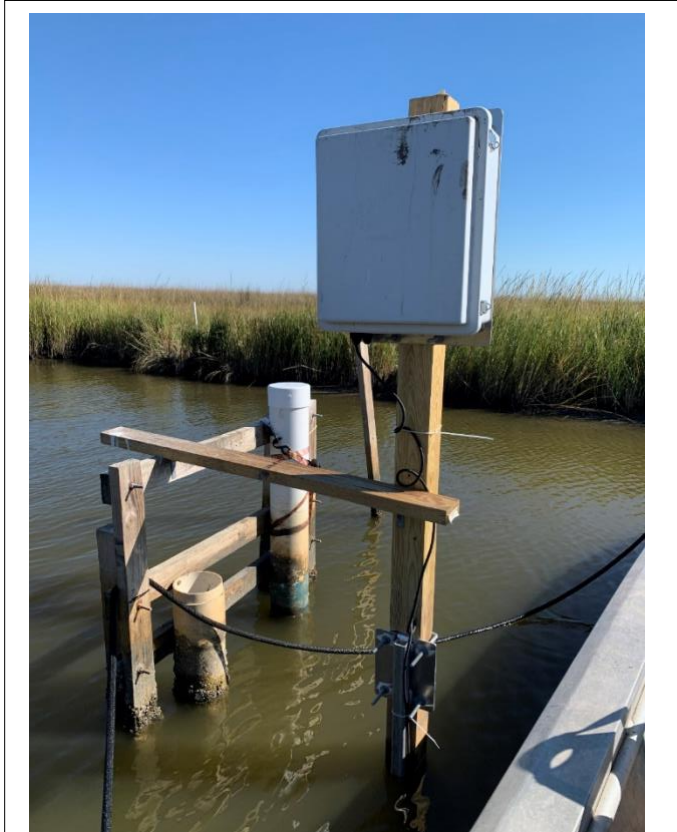
Figure 6. Lateral flux station located at the salt marsh site. The acoustic doppler profiler (ADP), YSI, EXO2 multiparameter water quality sonde and the Pro-Oceanus dissolved CO 2 data logger are mounted on the platform.
